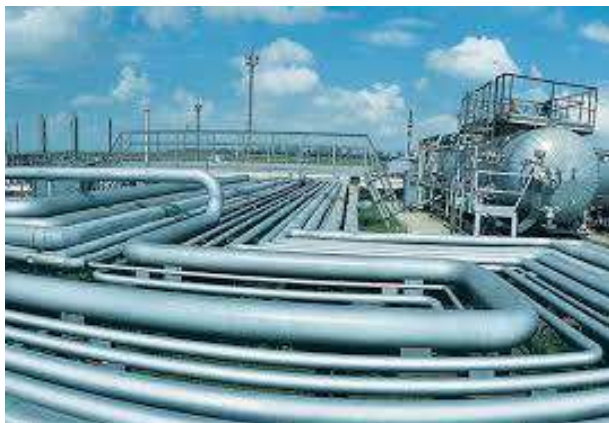
Trans-Saharan Gas Pipeline ndlink.org
